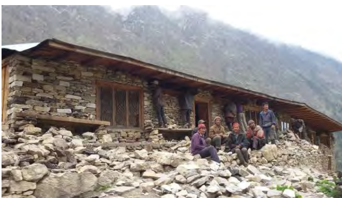
b) A stone house under remediation in the higher Himalayan region (source: Subash)
