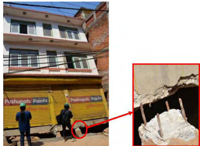
Photo 4: Collapse of a 3 storied RC (poor ductile detailing) Building
