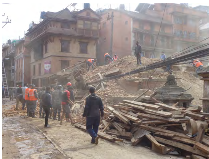
Community and armed forces helping salvage from collapsed temple in Patan © Kai Weise
