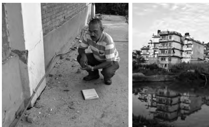
a) Ejecta from underneath the Fisheries Building b) Eastward view of tilted buildings near fisheries facility
