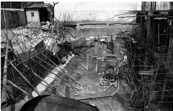
a) Northward view of the coseismic shoring failure at Kamaladi
