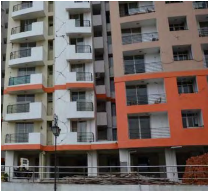
Photo 8: Diagonal cracks in the masonry infill walls
