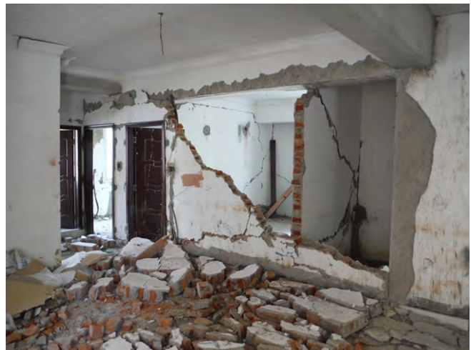
h) Diagonal tension failure and toppling of partition walls in a multi-storey RC frame building.
