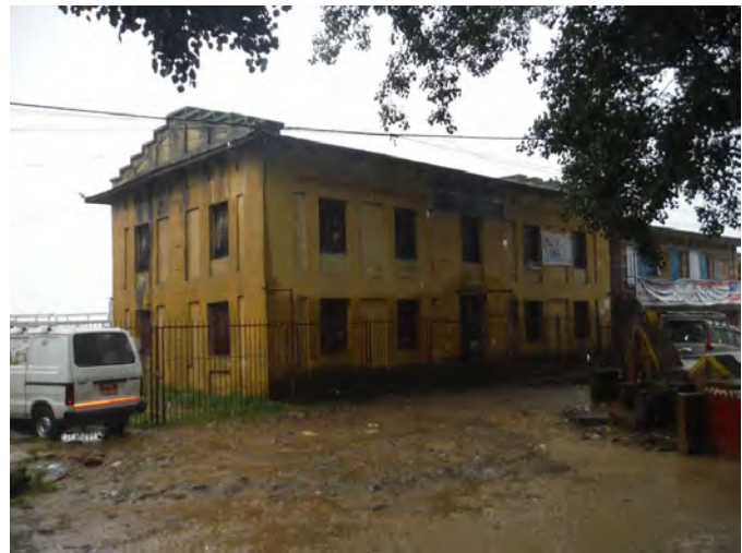
Figure 11: A strengthened brick masonry building in mud mortar (Kathmandu valley), the building survived without any damage.
