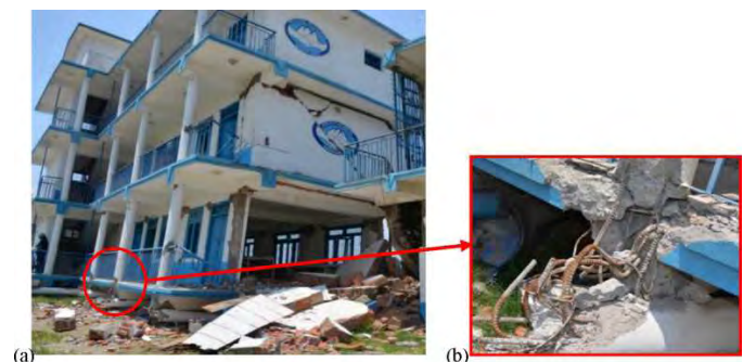
Photo 6: (a) Collapsed building (b) Shear failure of columns.
