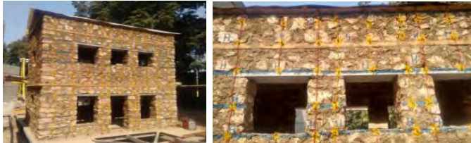
Fig 6 B - 2 1/2 story test model complete with all wire and WWM reinforcement. Yellow indicates GI, red indicates Aluminum, and blue indicates WWM strap band
