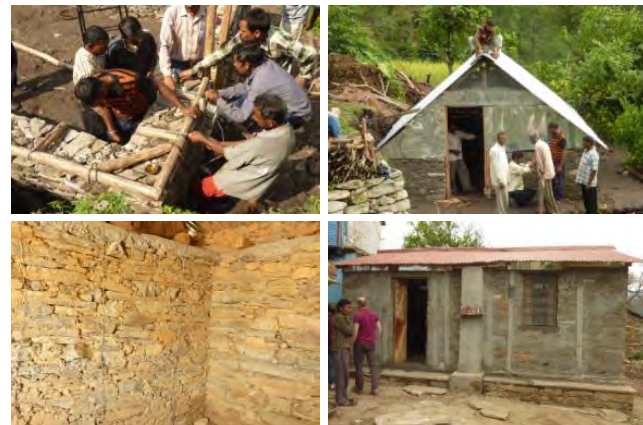
Fig 3 – Houses with GI wire containment reinforcement and wooden wallplate in Uttarakhand state after 2013 Himalayan Tsunami
