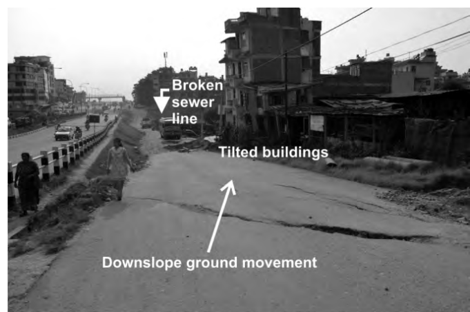
a) Westward view towards the Manohara river at Lokanthali ground failure site
