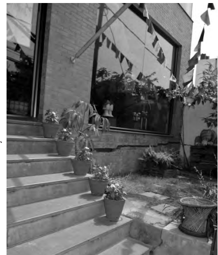
b) Westward view of damaged facade of the Sherpa Adventure Gear building due to shoring failure next door
