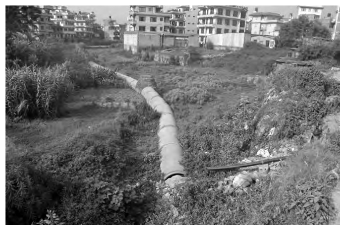
b) Northward view of the broken sewer line along the Manohara
