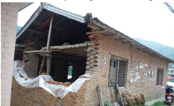
A brick masonry building with toppled wall.
