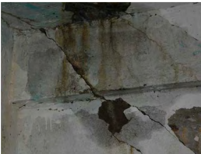
Photo 9: Diagonal shear failure of a beam
