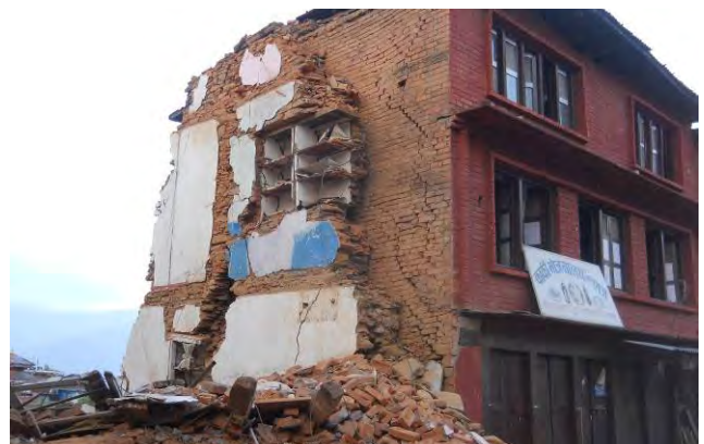
b) Brick in mud mortar, note a lack of positive connections between return walls.
