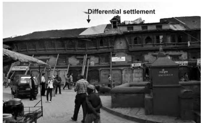
b) Southward view of a damaged unreinforced masonry structure west of Bhaktapur Durbar Square
