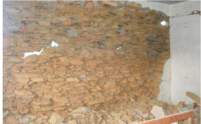
a) Delamination of stone masonry infill wall in a RC frame building.
