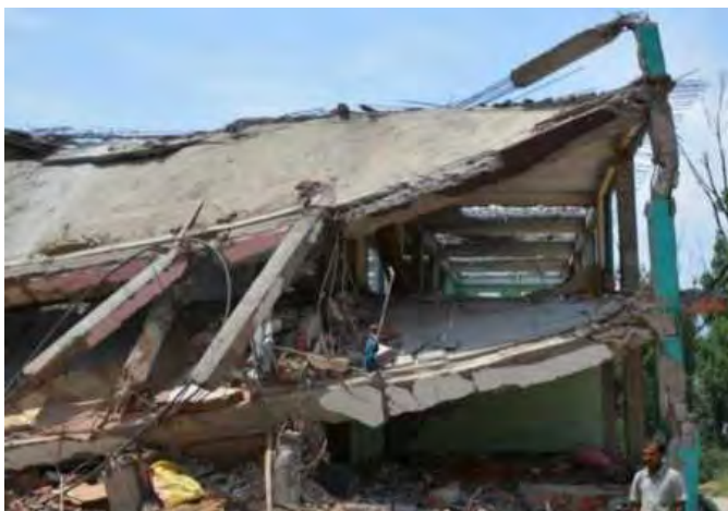
Photo 1: Collapsed RC frame building in Sitapaila
