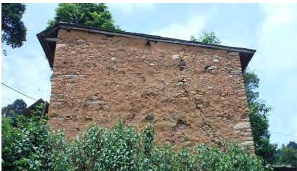
A stone masonry building with nominal damage.
