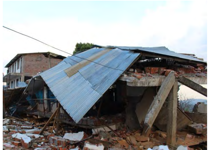
g) Disintegration of upper story.
