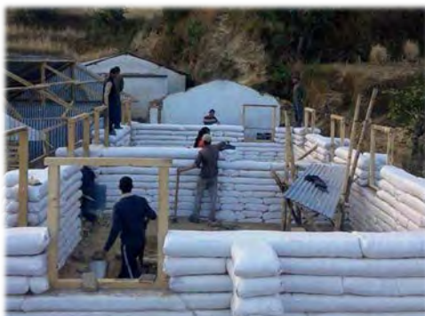
Figure 1: Earthbag Construction in Makwanpur, built by Good Earth Nepal (Good Earth Nepal, 2015).
