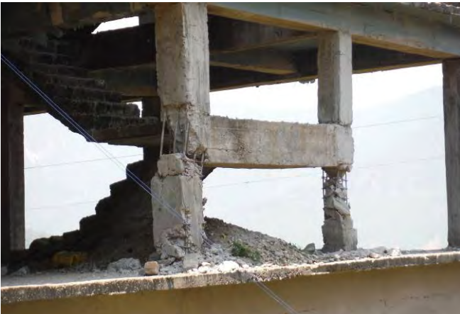
e) A damaged RC frame building (note lack of stirrups in the joint)
