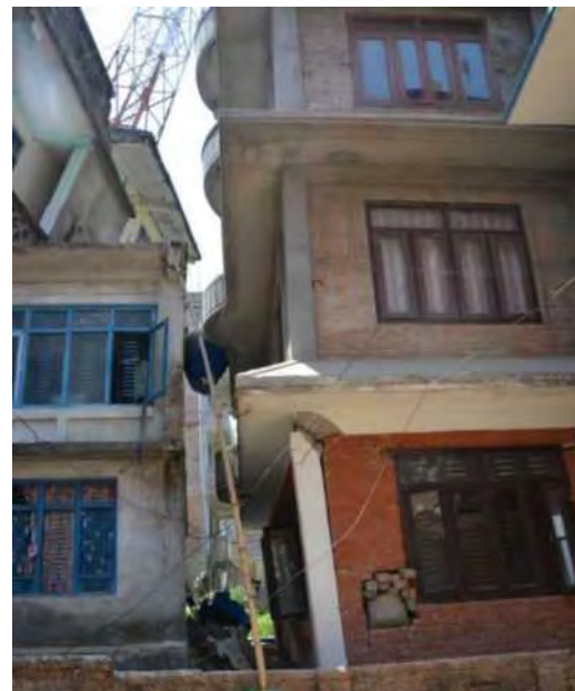
Photo 5: Damage to the first story of the 3 storied building
