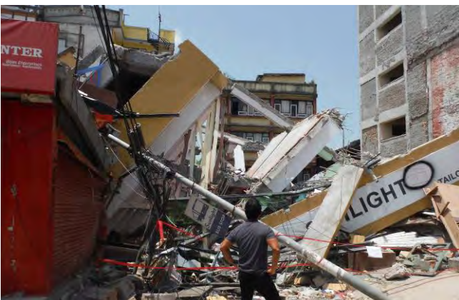
f) A destroyed RC frame building, note anchor failure of beam bars.
